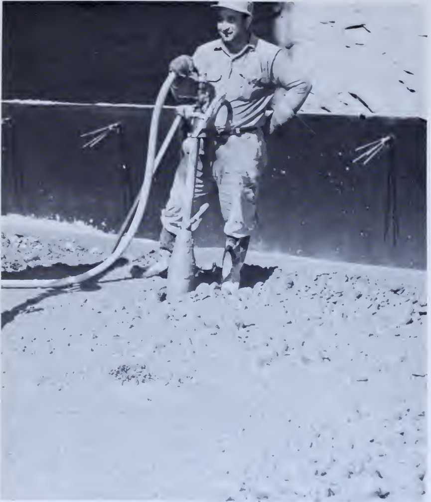
Figure 140.—Concrete after proper consolidation. Note that workman stands on concrete despite its appearance of wetness. P557-420-08212.
